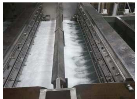
Chemical processing tank in an SKF coating facility
