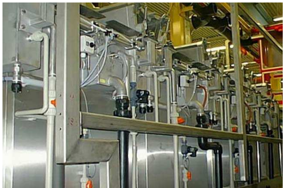
Phosphating plant at SKF
