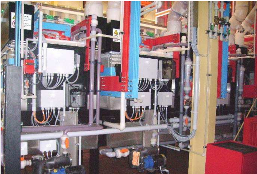
Galvanic coating plant at SKF
