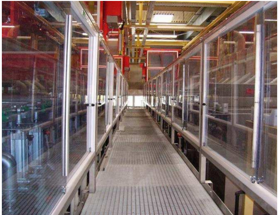
Coating plant at SKF Schweinfurt, Germany
